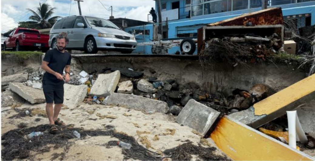
Concrete and other debris resulting from intense winds and waves sustained during Hurricane Fiona
